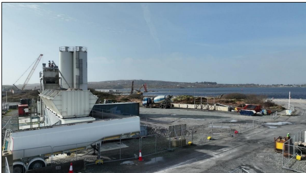
Figure 24: Photograph of the mobile Concrete Batching Plant and water storage tank.
